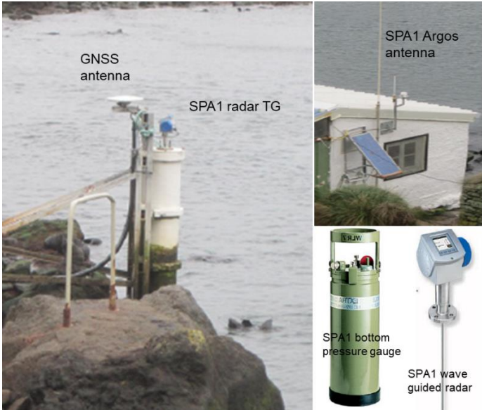
Figure 6 : Saint-Paul SPA1 station in 2014 with the stilling tube hosting the bottom pressure gauge (SPA_BPR), the wave guided radar gauge (SPA1_RDR) and the GNSS antenna; ARGOS antenna is set-up on the side of the cabin (Adapted from Nivmer report photos)
